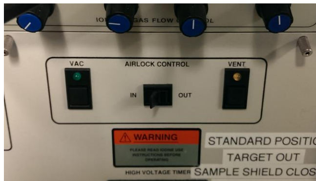
Figure 6. Close-up of Airlock Control
